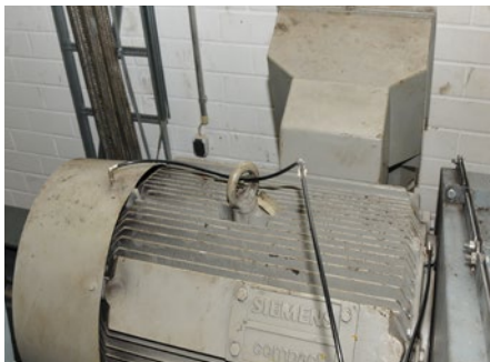
Lubricant supply on the fan drive
