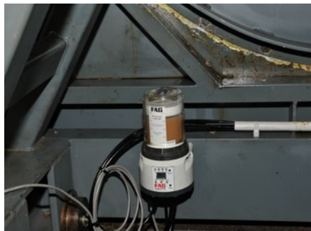
FAG CONCEPT8 lubricant system at the base of the fan housing
